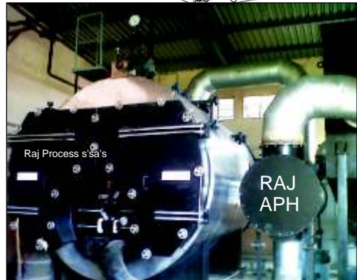
Husk Fired Boiler
